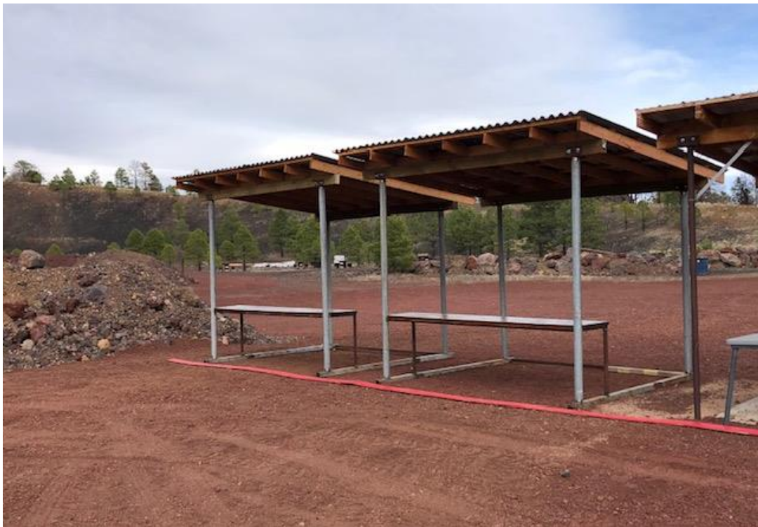
The framed and now roofed new Pistol ramadas on the main range. Picture by Keith Heimes.
