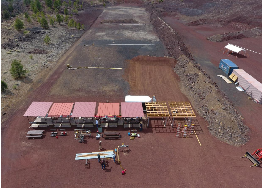
Aerial view showing the freshly groomed range surface and impact berm, and the newly framed Pistol ramadas. Picture by Nate Hedges.
